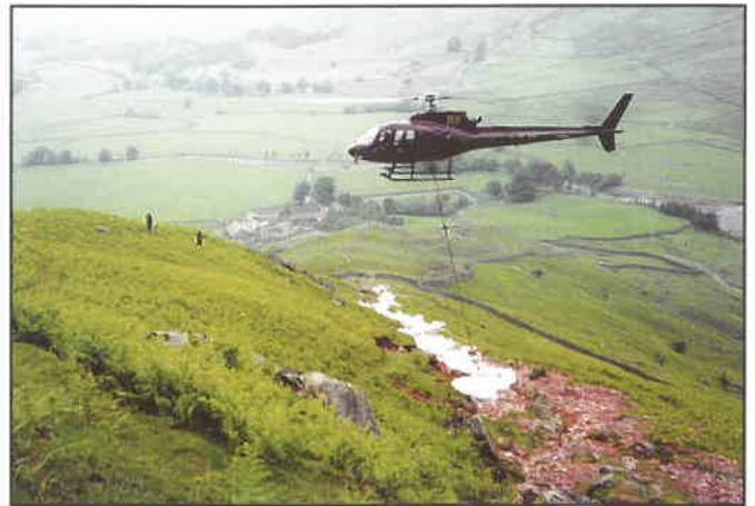
Delivering Victorian footpath repair techniques by means of modern transportation - using the best of both worlds to build a path for the future.
