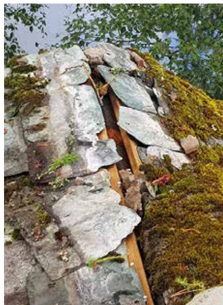
Lightning Strike Damage to Lodge 47 Roof
